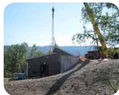
Follo fjernvarme (district heating) Follo Fjernvarme's pellet-fired heating plant in Ski will eventually become part of a major district heating grid in Ski.
