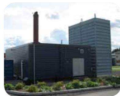
Oplandske Bioenergi's wood chip-fired bio-plant Oplandske Bioenergi's wood chip-fired bio-plant in Bagn delivers heat to municipal users in Sør-Aurdal municipality.
